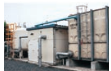
Industrial Wastewater Treatment System
