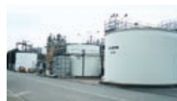
Activated Sludge Treatment System for Waste Liquids
