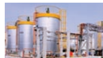
Recycling System for Wastewater and Sludge
