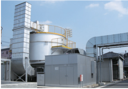
Noda Works of Hitachi Kasei Polymer Co., Ltd. introduced thermal rotating exhaust processing equipment and reduced VOC emissions by 95.7% compared with 2000 levels.
