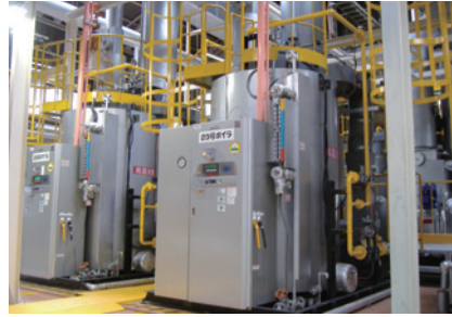
The Shimodate Works laid pipelines for natural gas and converted from heavy oil fuels to natural gas for through flow boilers.
