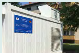
The exterior of the system in Speyer
